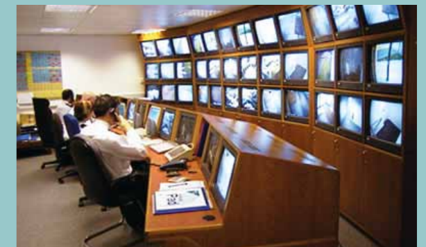
Security Systems / Control Room
